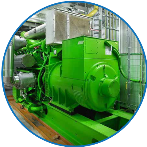
Combined Heat and Power unit (Source: Energuide)
